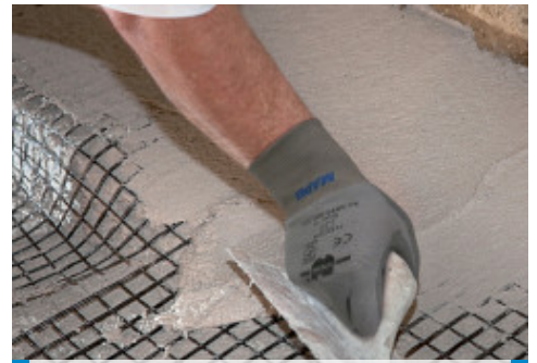
Application of the second layer of Planitop HDM Restauro by trowel on the outer face of a vaulted ceiling to cover the Mapegrid G 220 with an even coat
