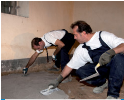
Application of the first layer of Planitop HDM Restauro by trowel on the outer face of a vaulted
