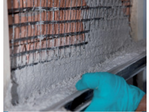
Application of Planitop HDM Restauro system with Mapegrid G 220 on a brick wall
