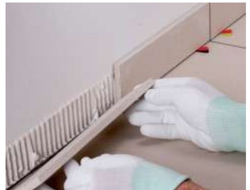
Apply the skirting around the room without letting it come into direct contact with the floor
