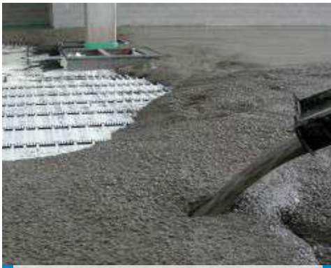
Pouring concrete with the addition of Mapefibre NS18 to counter plastic shrinkage
